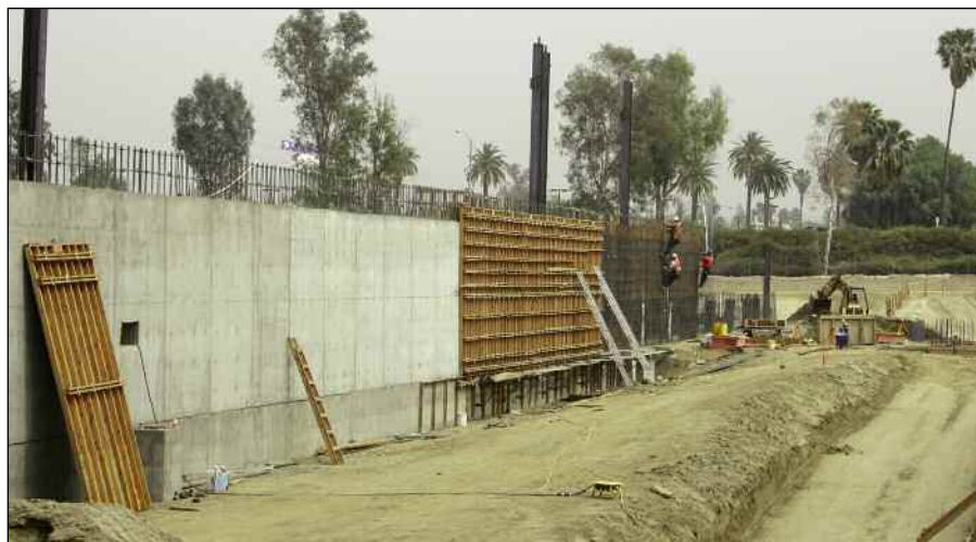
Construction has now begun on the Centennial Complex. This picture, taken March 20, shows the beginnings of the south wall.
