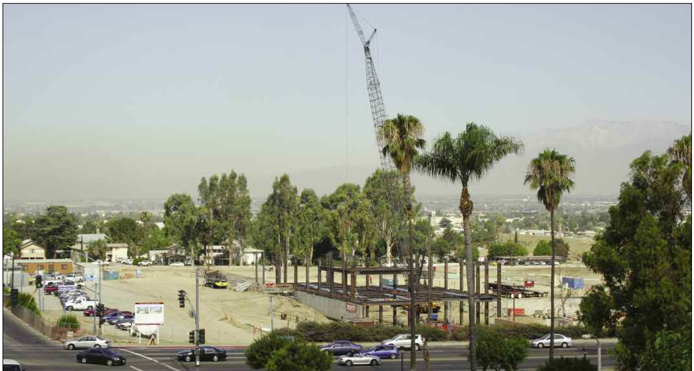
Steel beams—the skeleton of the new Centennial Complex structure—give hint of the presence the new building will have.
