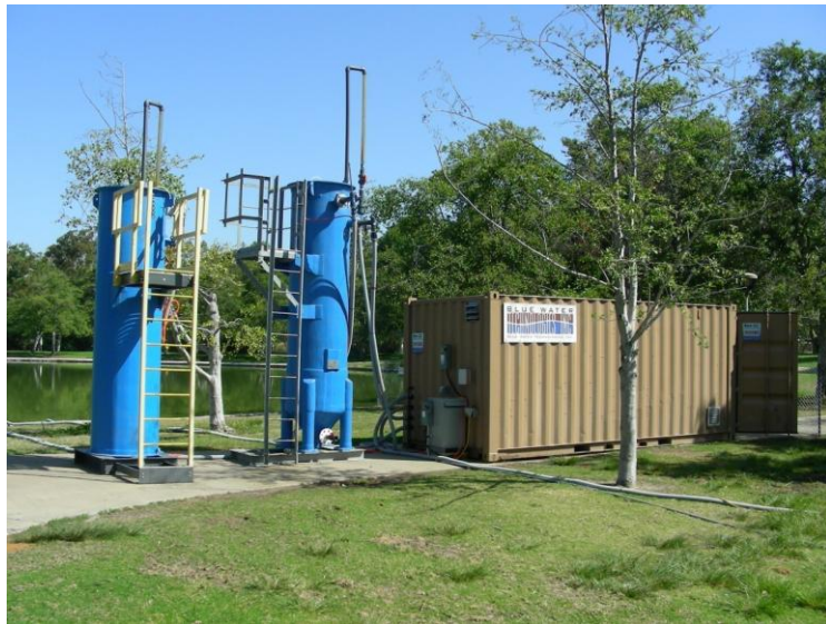
Fig. 3.1. Temporary Blue Pro™ water treatment facility at Mason Lake, April 2008. In a permanent facility, the sand towers can be embedded in the ground, and the trailer can either be camouflaged or decorated as an attraction for public education.
