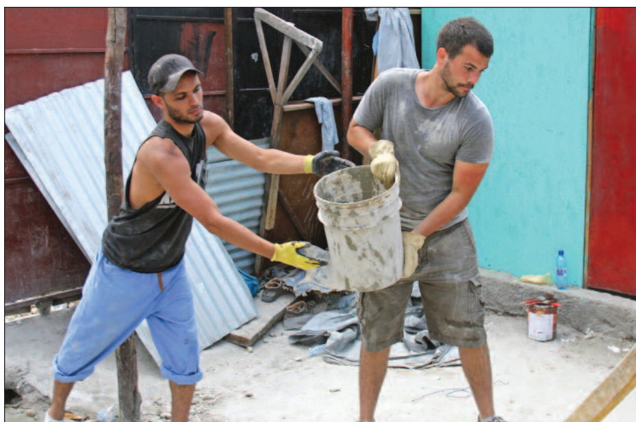
The cement bucket line for new roof columns at one of the orphanages gets its muscle from Alex Cabrera and Trevor Lohman, physical therapy students.
