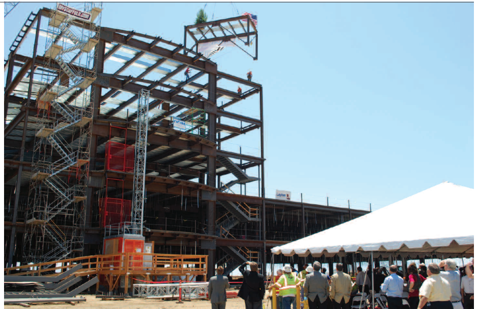
A crowd watches Thursday, May 21, as a construction crane hoists the last piece of steel beam for the new Loma Linda University Medical Center–Murrieta.
