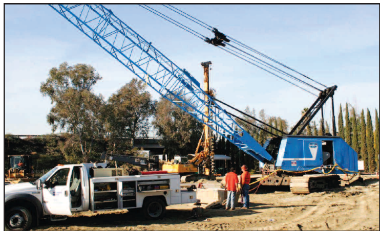
Construction workers examine the site where a new 6,000,000-gallon chilled water storage tank will be built. When completed, the behemoth structure will store chilled water used to cool buildings and equipment all over campus. The Anderson Street overpass is seen behind the trees in the center of the picture.
