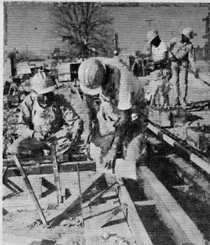
—Staff photo WORKMEN SPEED CONSTRUCTION on a new substation for the Southern California Edison Company at Mountain View Avenue and Redlands Boulevard. The unit is being erected because of anticipated increase in demand for electrical service when the University's Medical Center is completed.
