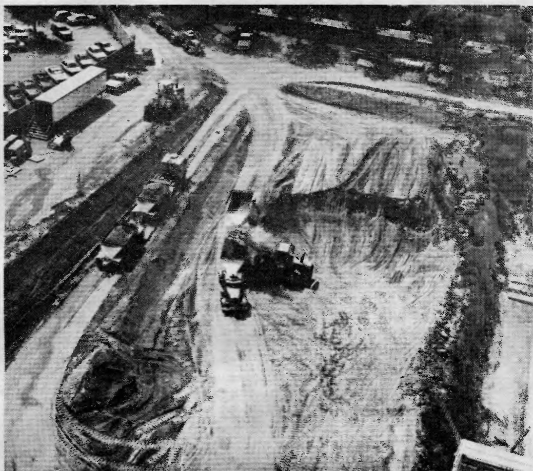
Earth-moving equipment has begun to dig out the site of the new wing that will house the proton-beam accelerator. The new facility, on the southeast side of the Medical Center, is expected to be completed in two years.
