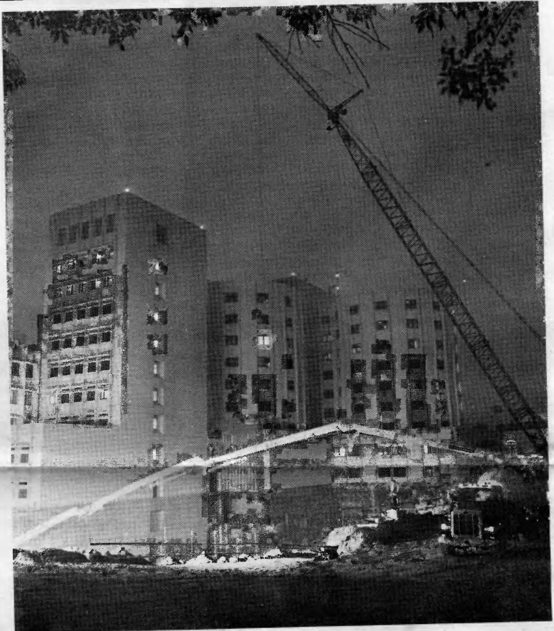
Beginning at 5 a.m. on November 7, trucks loaded with concrete began arriving at the construction site of the world's first hospital-based proton accelerator for the treatment of cancer at Loma Linda University Medical Center. By 7 p.m., the trucks had dumped 2,800 tons of concrete for the building's foundation.
