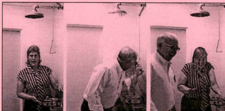
Nancy Pulliam, director of infection control, was explaining the emergency shower system when Chuck Yetter, assistant director of maintenance, decided to give her a helping (?) hand! 5
