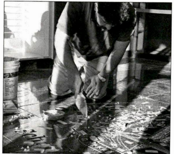
A worker installs the brass and marble School of Dentistry seal in the School's entrance. The project is one of many funded by generous donors.
