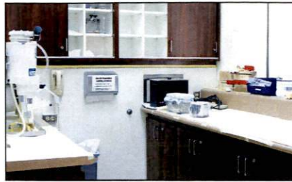
The South Clinic has had a face lift. Dental supply staff installed new cabinets, sink, and window in the supply room, and painted room 2202.
