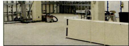
The 1140 laboratory remodel has started. It is slated to be finished the end of this month.
