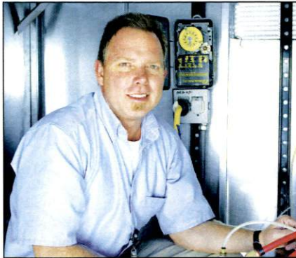
Stan Lillard installs the new water system in the endodontic clinic. Plumbing and water systems have been installed throughout the School.
